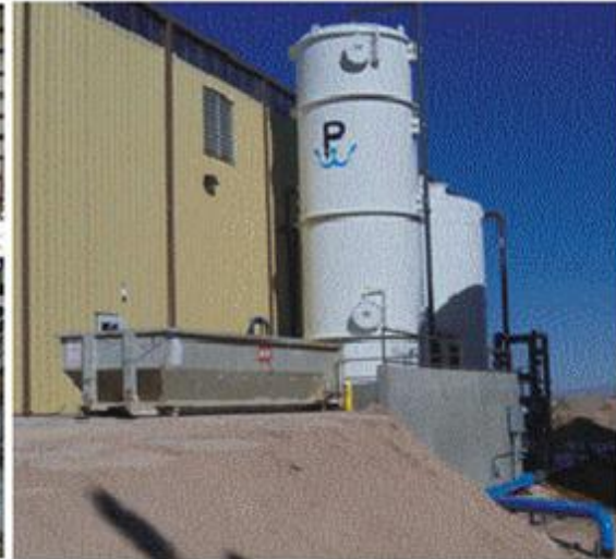
Vacuum Clarifier - Secondary Separation
